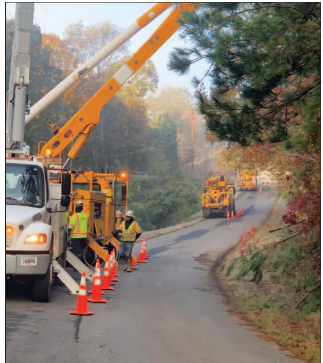
CEMC workers provide assistance to neighboring co-op Meriwether Lewis Electric Cooperative, which was also heavily impacted by the strong storm system.
