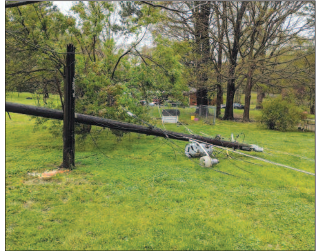
Major storms can cause damage to the power distribution system like this broken pole.
