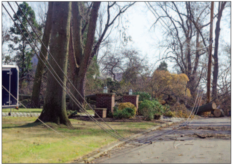
Downed power lines may still be live, even if you don't see sparks. Always keep your distance and report to your local co-op immediately.
